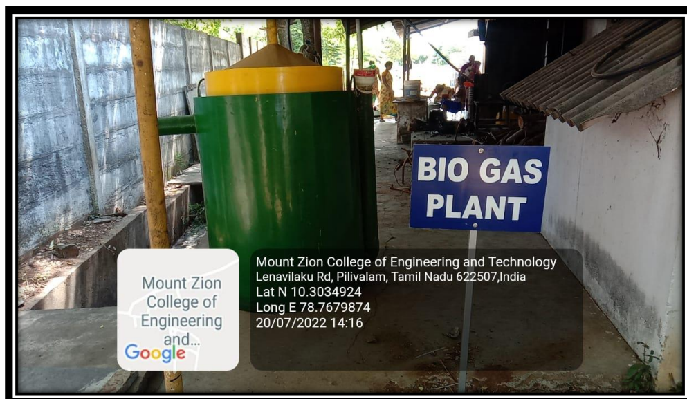
Bio gas plant located in the college kitchen
