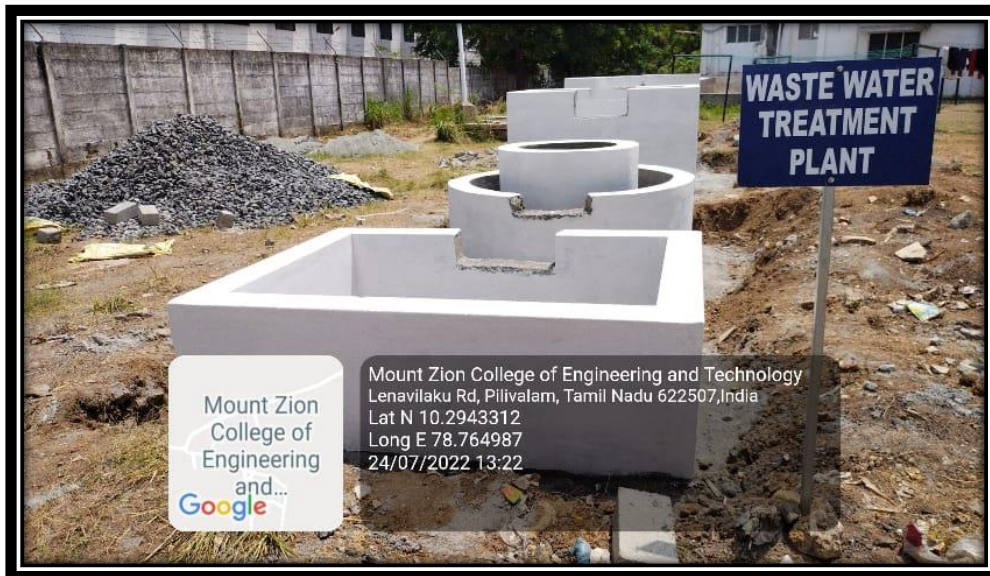
Wastewater treatment plant
