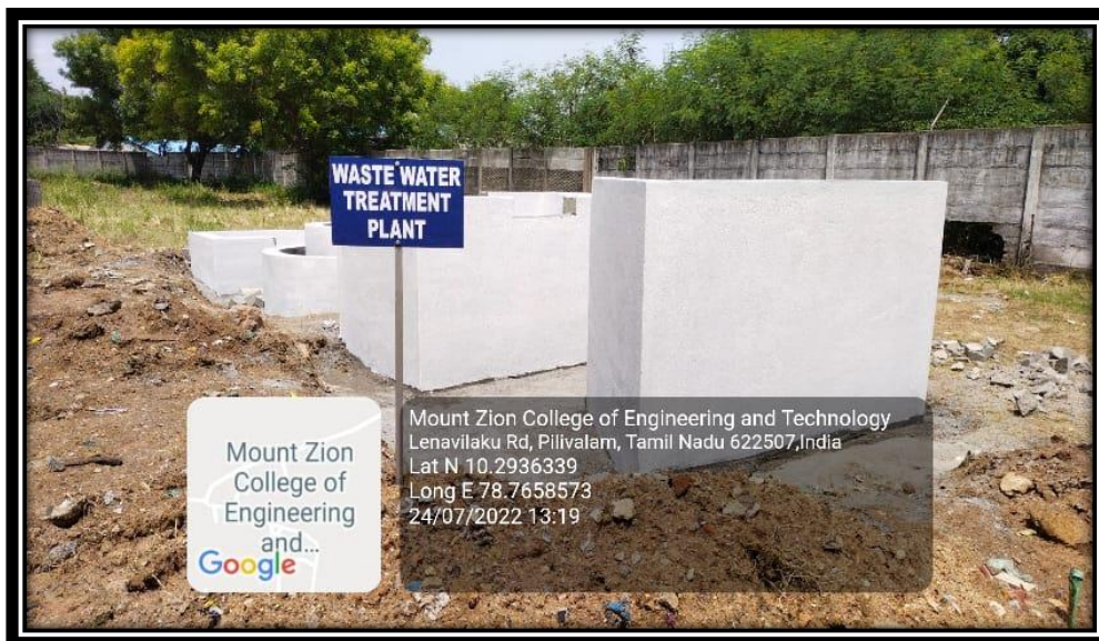
Waste water treatment plant
