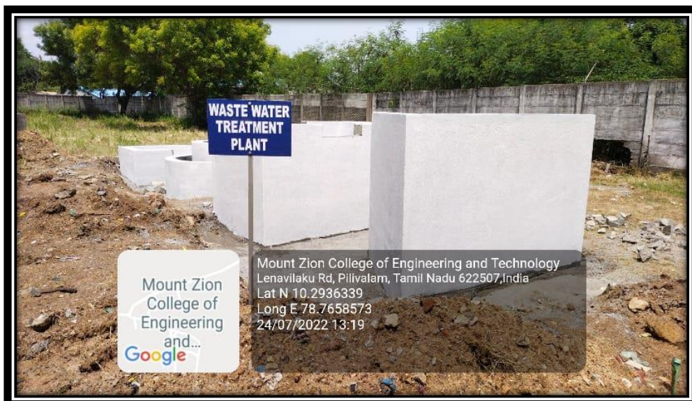
Wastewater treatment plant
